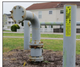
GOING, GOING ... VNG’s abandoned riser in the 4900 block, and one of Dominion Power’s damaged poles, 8100 block
