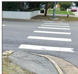
This is an example of non-compliant ADA ramps, at Bay Colony Drive.
